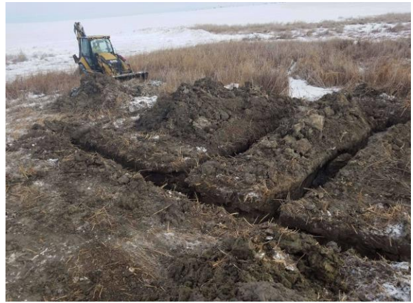
Photo #10 View of excavated trench grid pattern for dewatering and looking for flow patterns.
